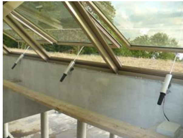
Fig. 4 Automatic openable windows, electric [5]
